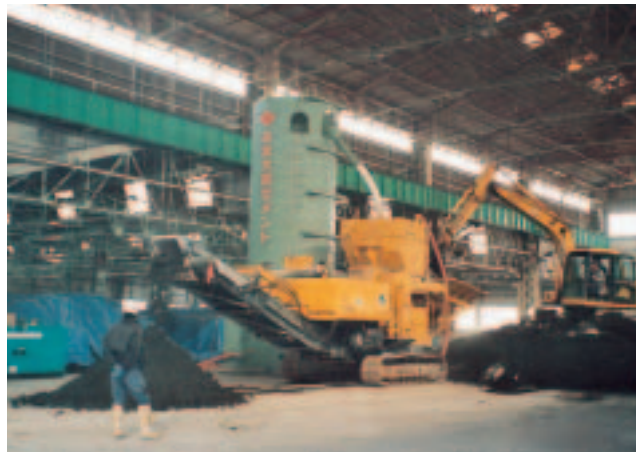
Example of decontamination operations for contaminated soil Rehabilitating soil contaminated with volatile organic compounds using a mobile soil stabilizer (BZ200 pictured)
