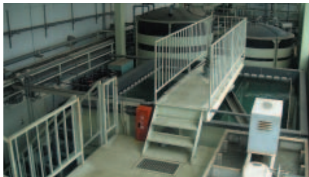
Wastewater treatment facilities
